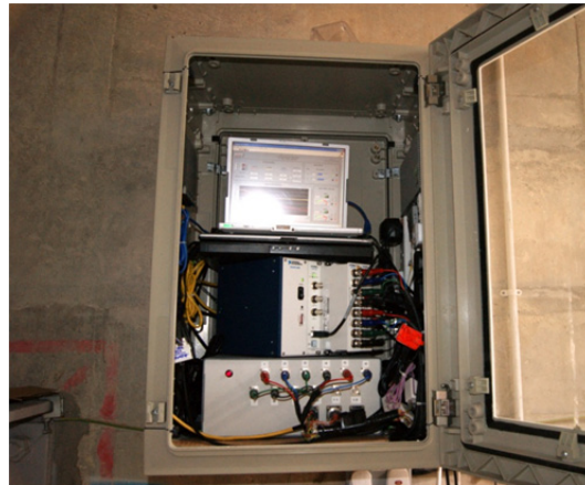
Figure 4.11: Unit containing Toughbook laptop, located in a control chamber.
