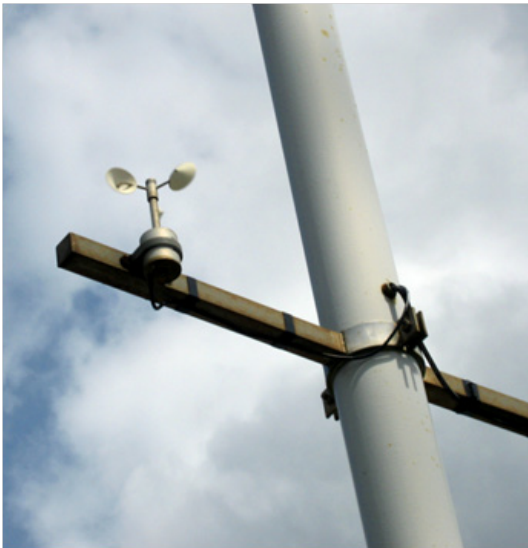
Figure 4.4: Anemometer located on a mast near the Saltash tower.
