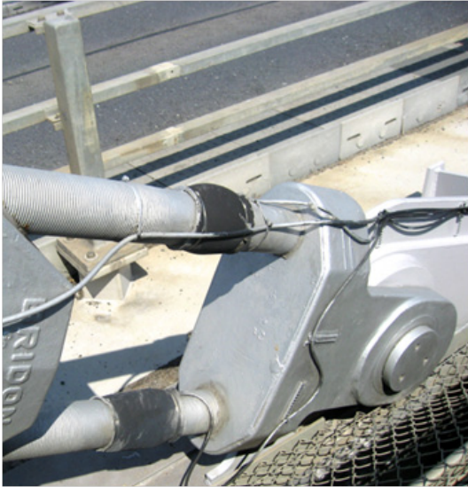
Figure 4.2: Strain gauges on a stay cable's tensioning bolts.
