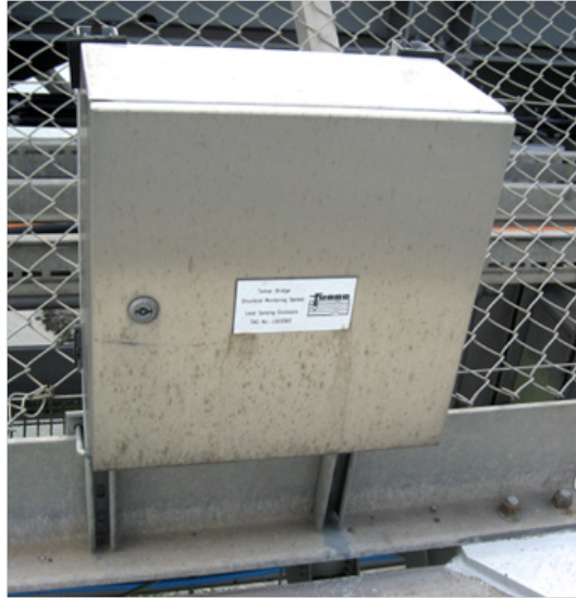
Figure 4.3: Box for a level sensor located on the bridge deck.
