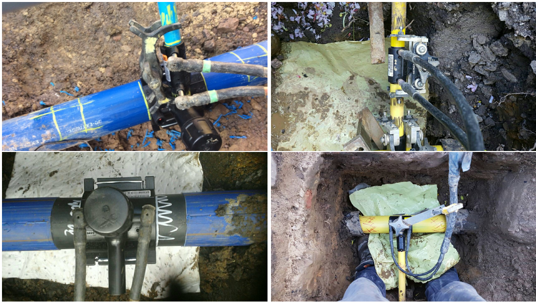
Fig. 1.3 Samples of the water and gas pipe images.
