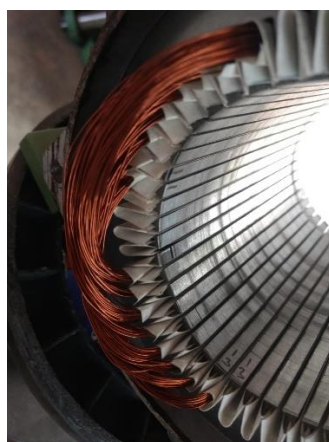
(b) Inserted coils
