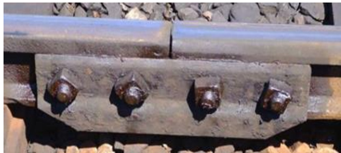
Figure 23. Rails connected by fishplates [16].
