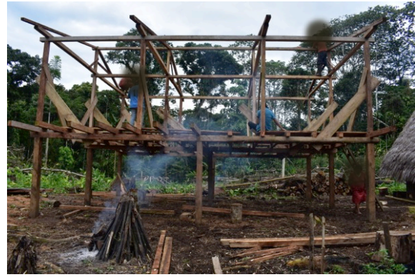
Picture 29 (right) the entire family contributing and working to build a new traditional house
