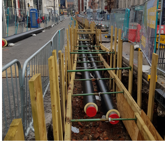
Figure 2.9: District heating pipelines (Leeds city centre).
