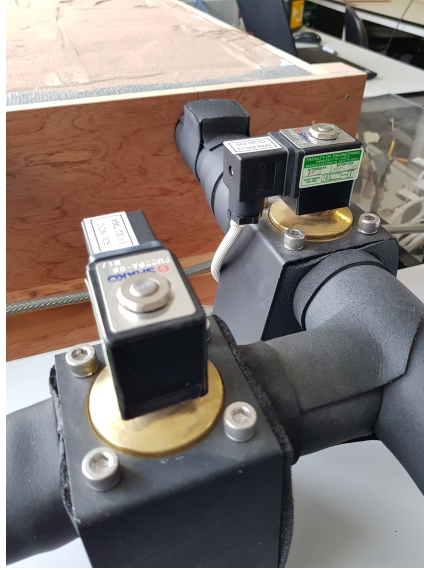
Figure 4.11: The brass solenoid valves arrangement in the test rig.
