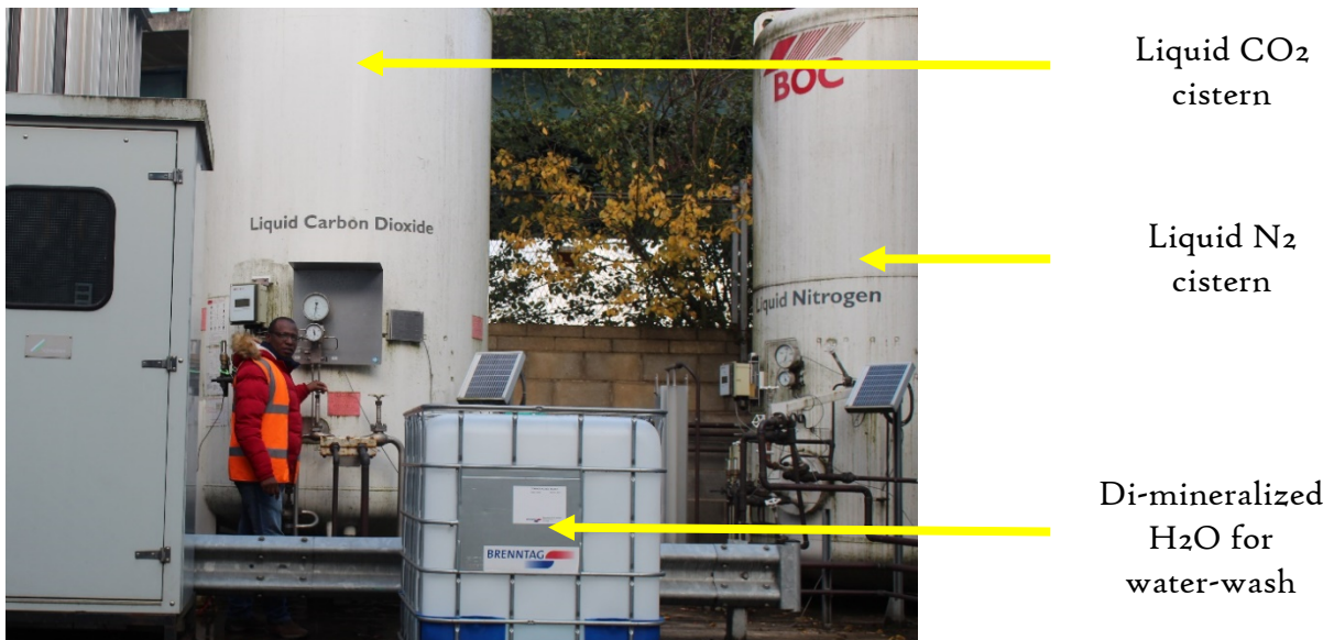
Fig. 3.8 Photograph of the gas storage facilities [110].
