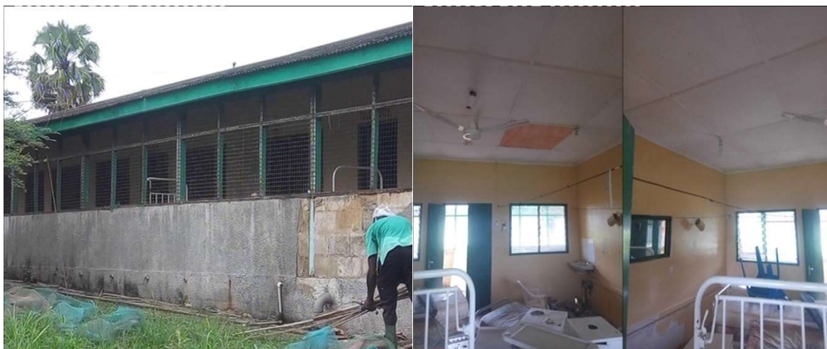
Pic 9.3 The state of the Antenatal ward at Mampong General Hospital Pre-reconstruction
