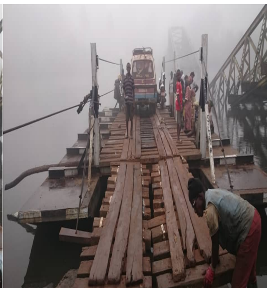
Fig. 14 This hardship of the journey was the result of a broken bridge that remained unrepaired for year Source: Author 2017.
