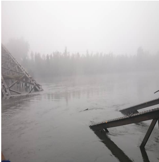
Fig. 21 Broken bridge hindering access to Bauya. Transportation is a major challenge, Mabang, Sierra Leone Source: Author 2017.
