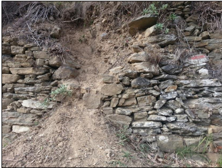
Fig. 3. Cinque Terre. A broken drystone terrace wall. Photograph by author.
