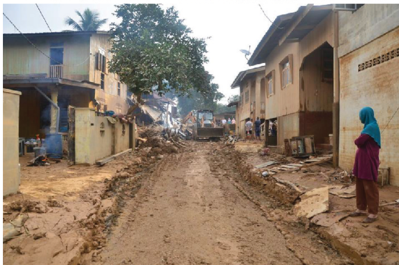
Figure 5.18 The excavator used to remove thick mud on the road (Source: bharian, 2015)
