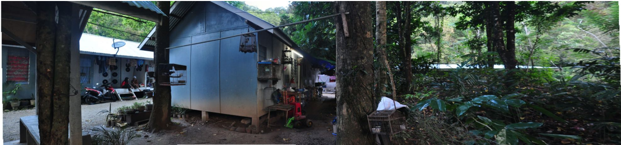
Figure 5.33 Watermark shows the level of floodwater raised during flooding, December 2015 (Nor Izura T., 2015).
