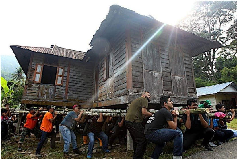
Figure 2.18 Traditional Malay house is designed portable responding to the local weather and context (Source: Malaymail, 2018)
