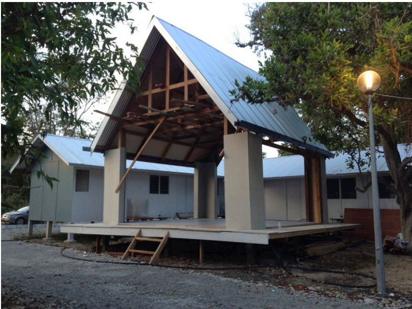
Figure 5.29: In progress: A multi-purpose space for the people to utilise as a prayer area, for discussions and meetings (Nor Izura T., 2015)
