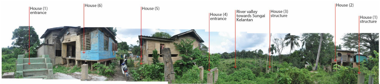
Figure 5.37: Post-flood view at Kampung Jalan Gaele taken from the alleyway. Kampung houses at this area were drifted away during the flood. Their house entrances and structures left at the site, marks the original location of their houses. Wild weeds and shrubs covered the areas. The residents in this area were not allowed to come back and rebuild their houses by the landlord. Therefore, they had to be displaced involuntarily. Taken on 16th December 2016 (Nor Izura T., 2015)
