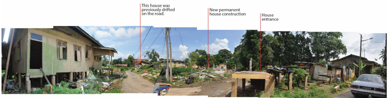
Figure 5.36: Post-flood view at Kampung Jalan Gaele. Watermarks from the flood can be seen clearly on the wall of the house (left). Taken on 16th December 2015 (Nor Izura T., 2015)
