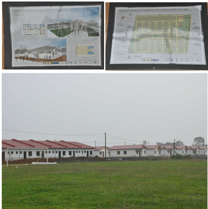
Figure 5.38 Permanent housing development for flood victims under construction in Kampung Telekung, 18 th December 2015 (Nor Izura T., 2015)
