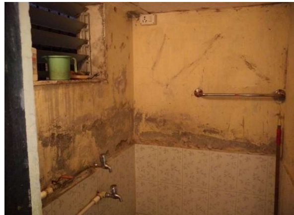
Figure 8-2 A picture showing faults in the construction (Source: author's own, 20 March 2016)
