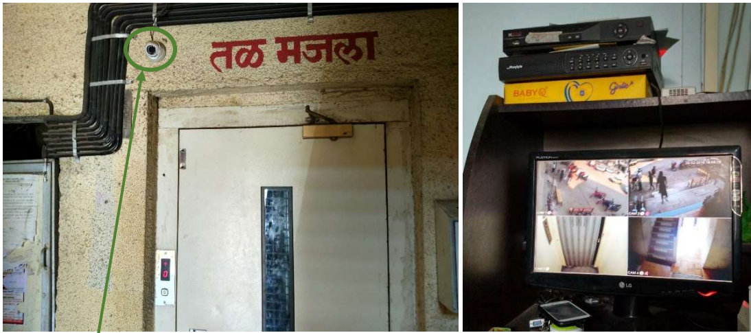
Figure 8-6 From left to right: Picture depicting the location of the CCTV Camera in the tower block (source: author's own, 19 th January 2016); Picture showing the CCTV camera main unit installed in a committee member's house (Source: author's own, 28 th February 2016)
