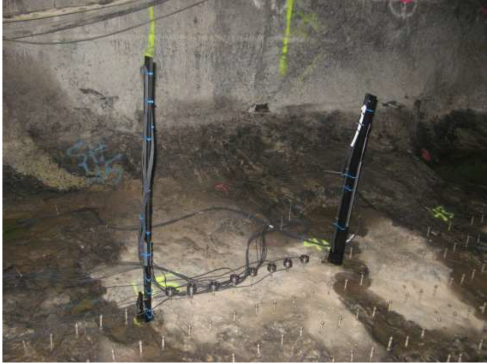
Figure C.4: Example survey during the EDZ study showing the setup of the borehole and surface frames. (Reyes-Montes & Flynn, 2015).
