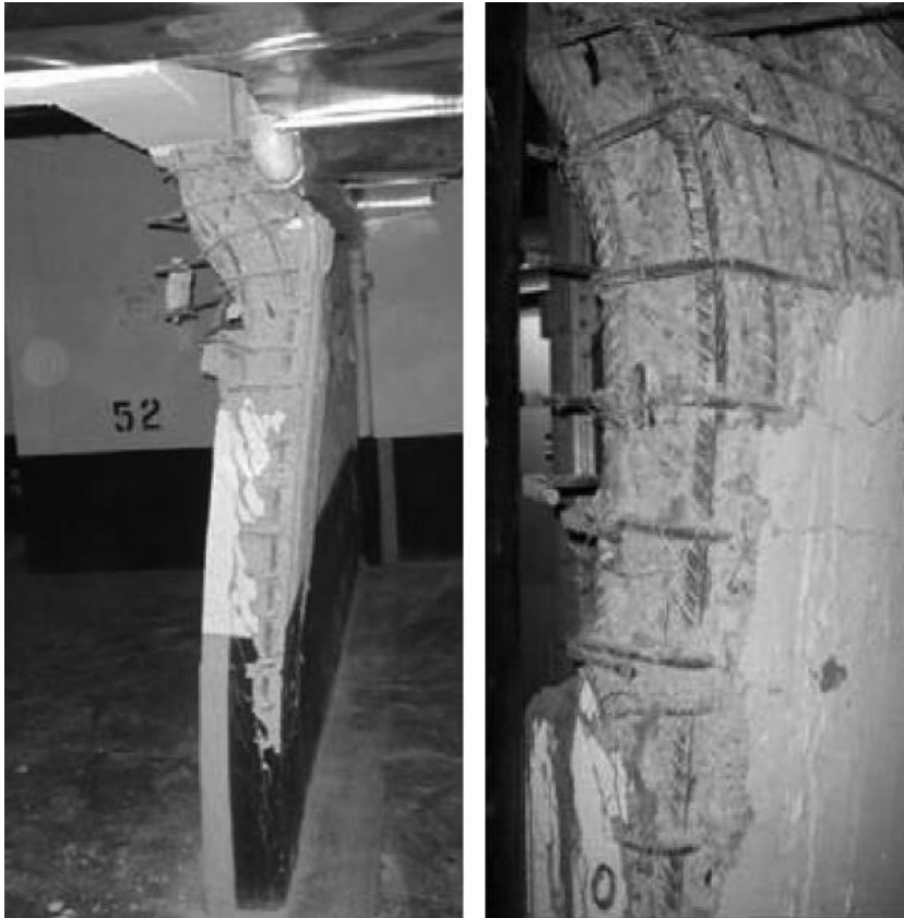
Figure 2.10. 2010 Chile M_w 8.8 Earthquake: Wall lateral buckling (after Wallace, 2012)
