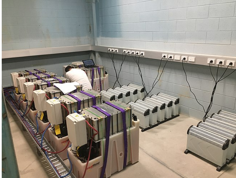
Figure 2.1: RedFlow Zn-Br 10kWh flow batteries in a performance testing lab
