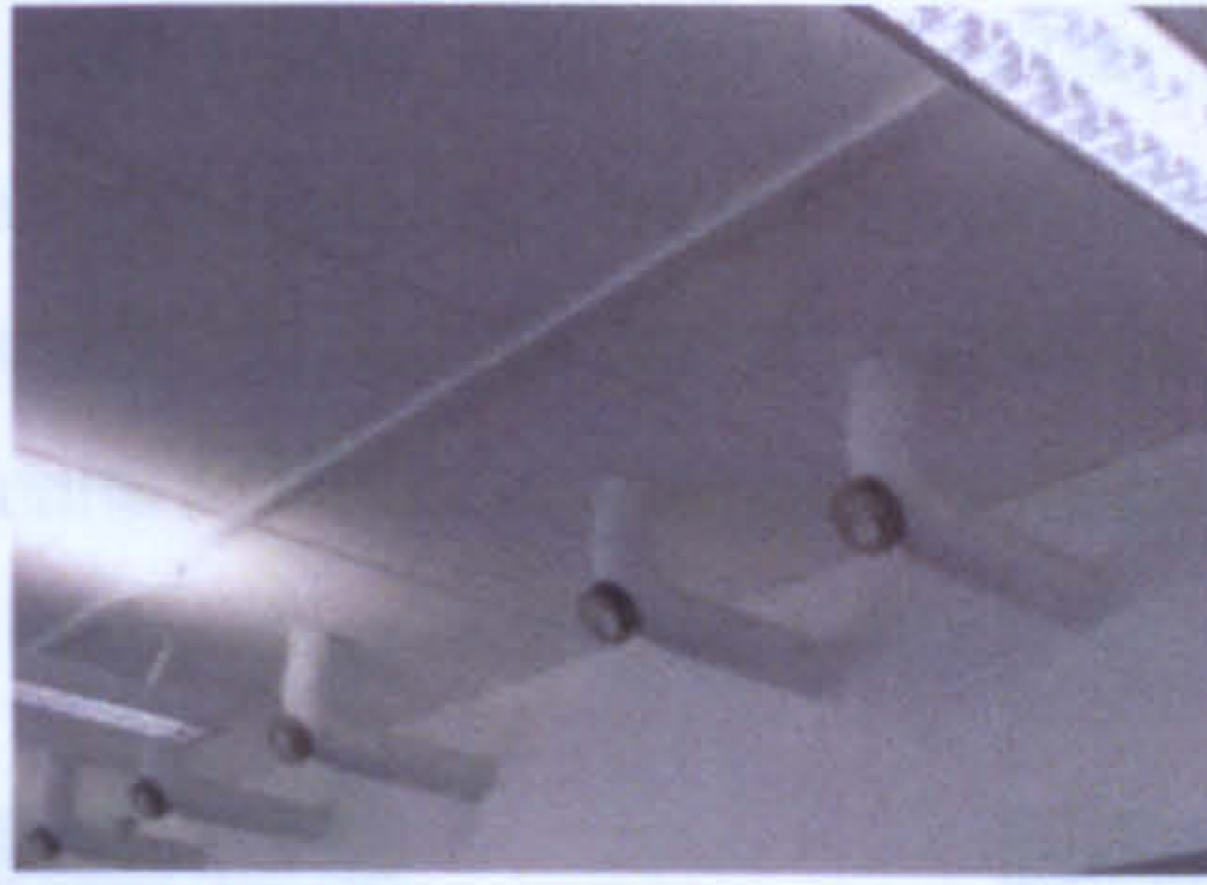
Figure 5-36: No extract vents within the cellular office
