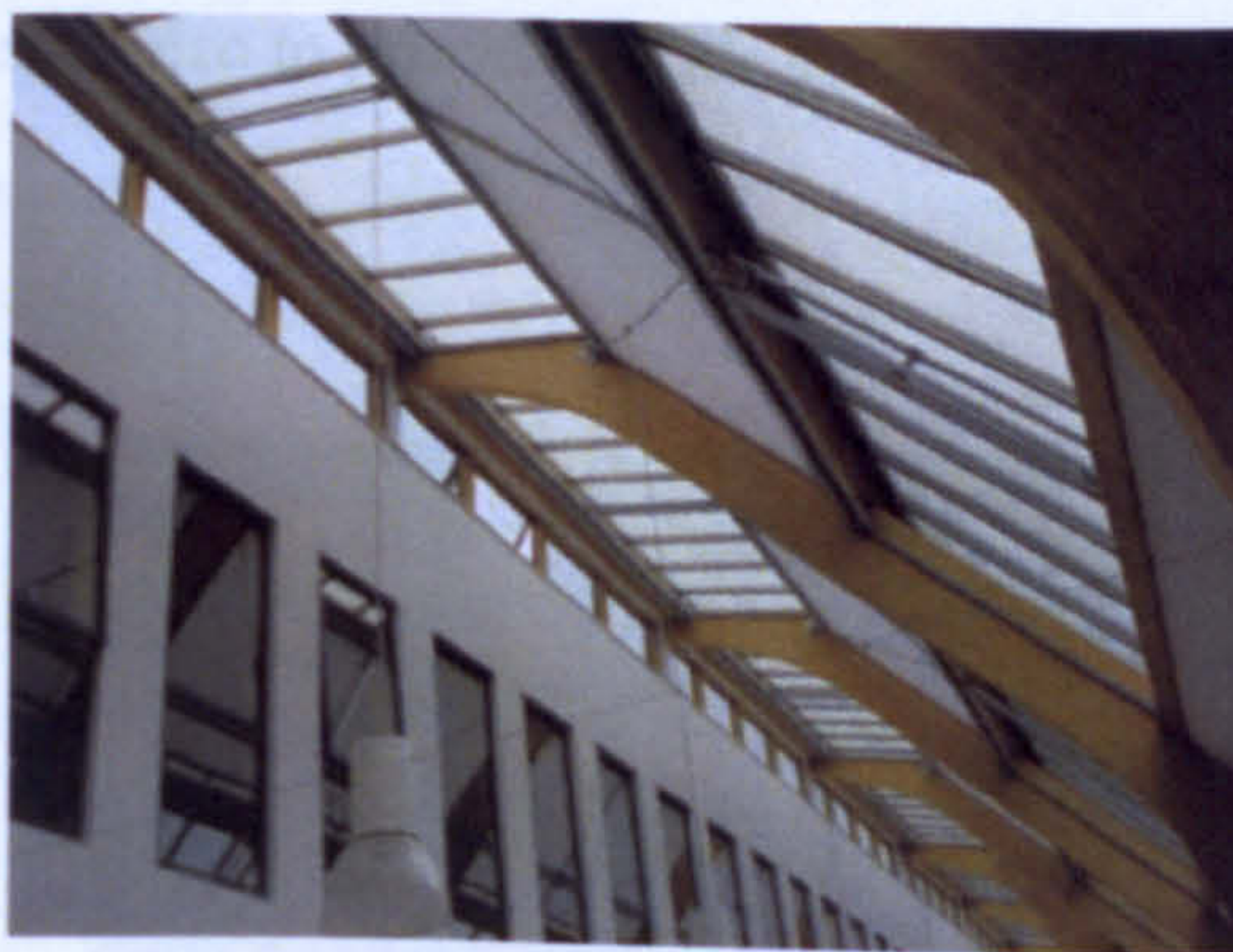
Figure 5-33: Broken actuators in the natural ventilation strategy within the atrium
