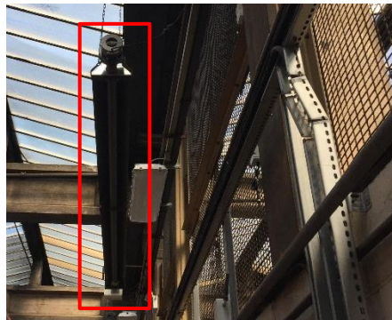
Figure 7.7 Ambirad radiative heaters in the repair shed of the Leeds depot
