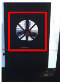
Figure 7.5 Roof fan in the repair shed of Neville Hill depot
