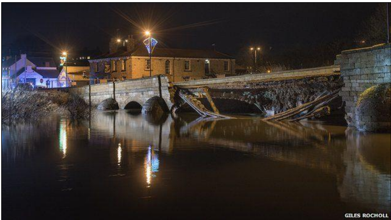
Figure 2.5. Collapsed section of a historic bridge in Tadcaster following heavy rainstorms during Storms Eva and Frank in December 2015. Copyright Giles Rocholl
