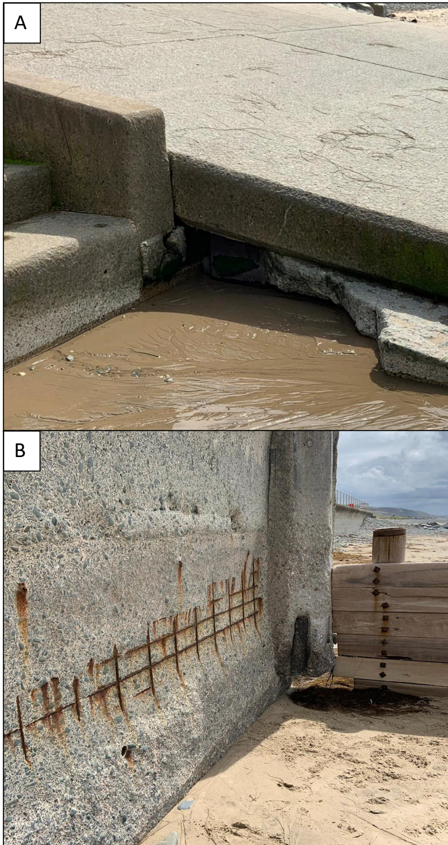
Figure 8.2 cont. Evidence of beach lowering and undermining of defences at the slipway (A) and sea wall (B) at Tywyn.
