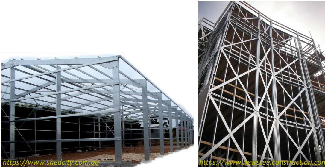
Fig. 1.1. Cold-formed steel (a) industrial structures with moment-resisting portal frames and (b) multi-storey residential building with stud wall system
