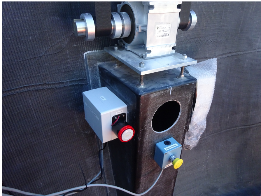
Figure 8.11: The Arduino box and yellow quick-close button in the GOTO dome, attached to the southern pillar under the dome drive. The cables run to the computer rack which is just off to the left of the photo.
