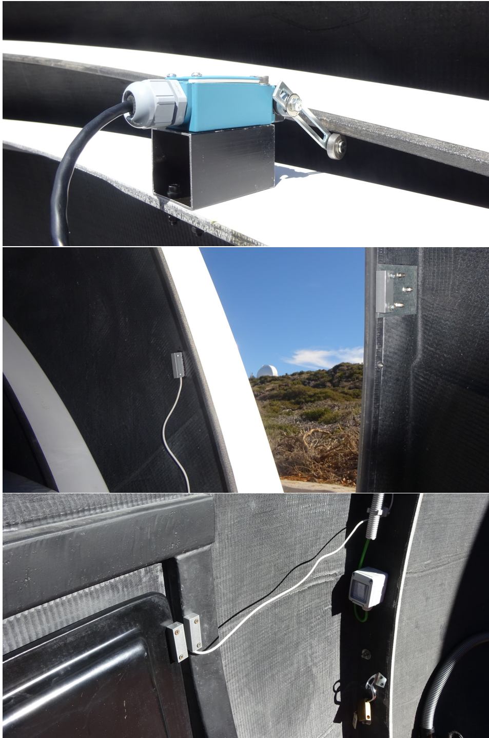
Figure 8.12: Additional sensors added to the dome. The top photo shows one of the two Honeywell limit switches added to the rim of the dome wall to detect when the dome is fully open, the middle photo shows magnetic switch added to the inner-most shutters to detect when the dome is fully closed, and the bottom photo shows the magnetic switch added to the dome hatch to detect when it is open.
