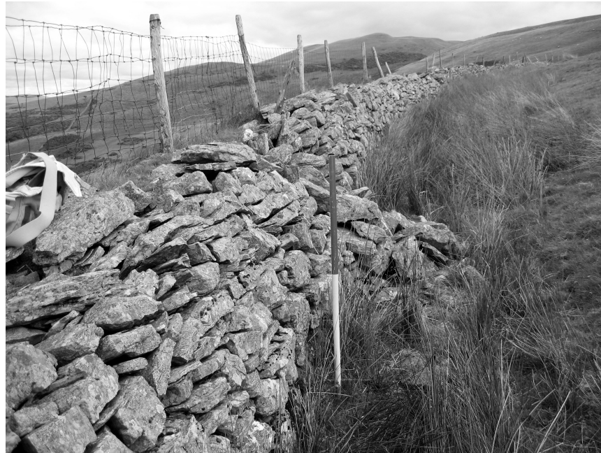
Figure 34: Looking north-west along the 'outside' face of the head-dyke near Fell Side.
