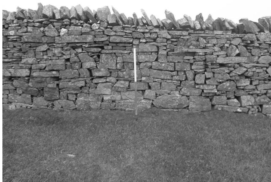
Figure 29: A wall with transverse capping in a good state of repair near Bramley Seat
