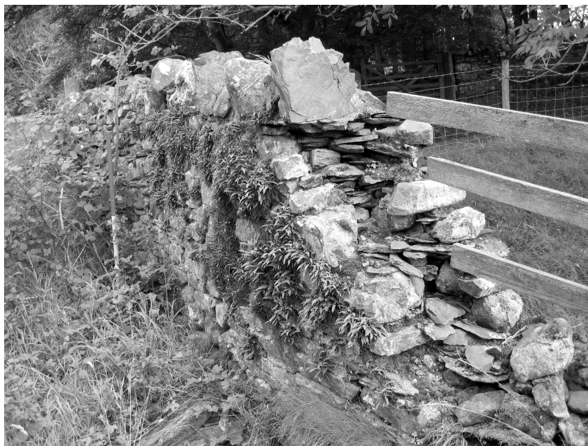
Figure 32: A wall constructed or repaired using mortar, with an inner core of slate and shale, on the road to Sosgill.
