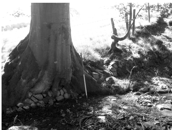
Figure 35: Wall overgrown by large ash tree.
