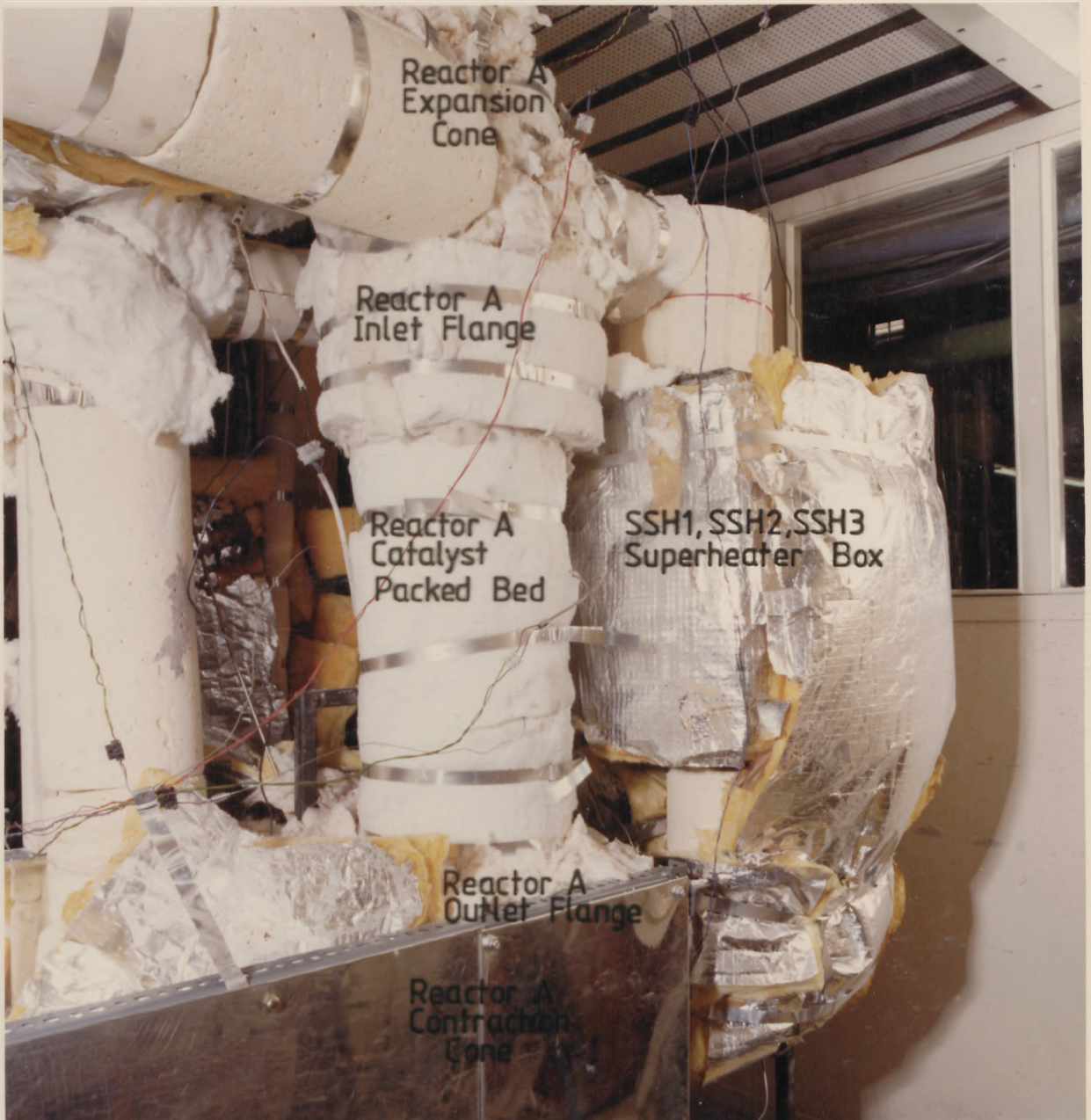
PLATE 2: Reactor A and the Superheater Box (Control Room)
