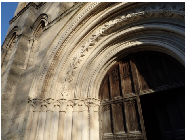
Figure 102: hot mixed and applied lime sheltercoat, St Mary's priory church, Old Malton, 2011
