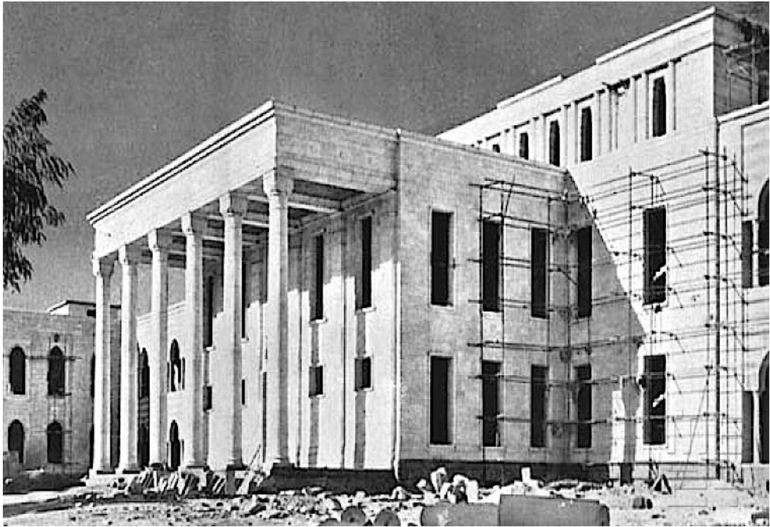
Figure 3-3: The Iraqi Parliament building, architect J.B. Cooper, Baghdad, under construction in 1957 and later transferring to the Ministry of Defence in 1959
