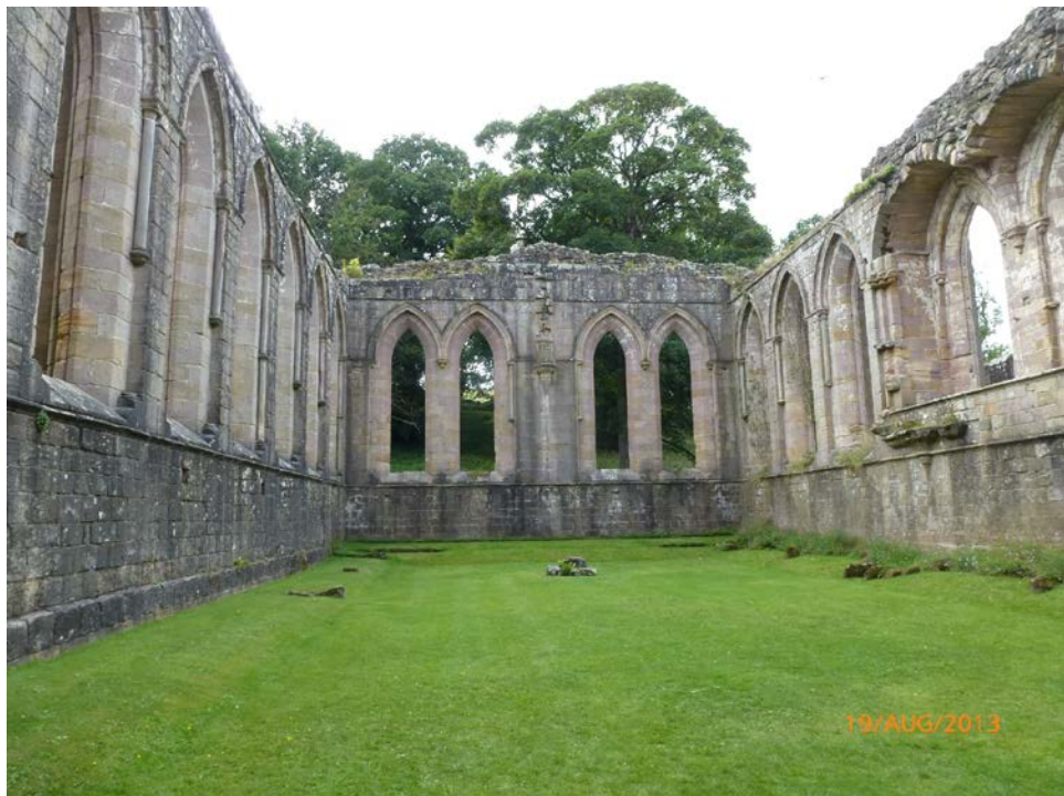
Figure 3i: The refectory was conserved with rough-racking, the built-up stones on the wall top at the far south end, and soft topping on the east and west elevations (These techniques were used by the Estate and the MPBW, respectively)
