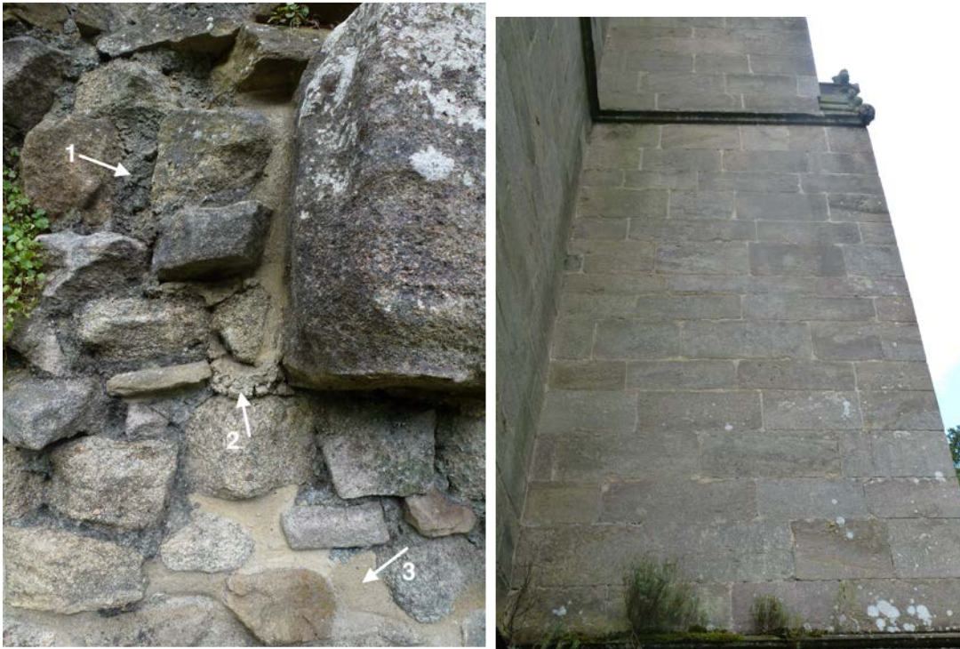
Figure 30: The guest house's array of unfinished neat cement pointing (1), untamped white cement (2), and wider, sandy joints (3) for comparison with the neater pointing of Huby's Tower
