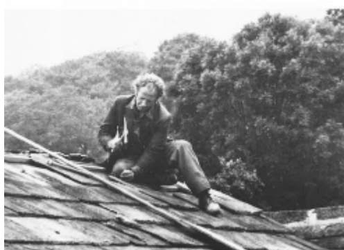
Figure 1b: Rees Morgan's (1981) photograph of a Yorkshire roofer 'us[ing] a slater's hammer to cut stone roof slates'
