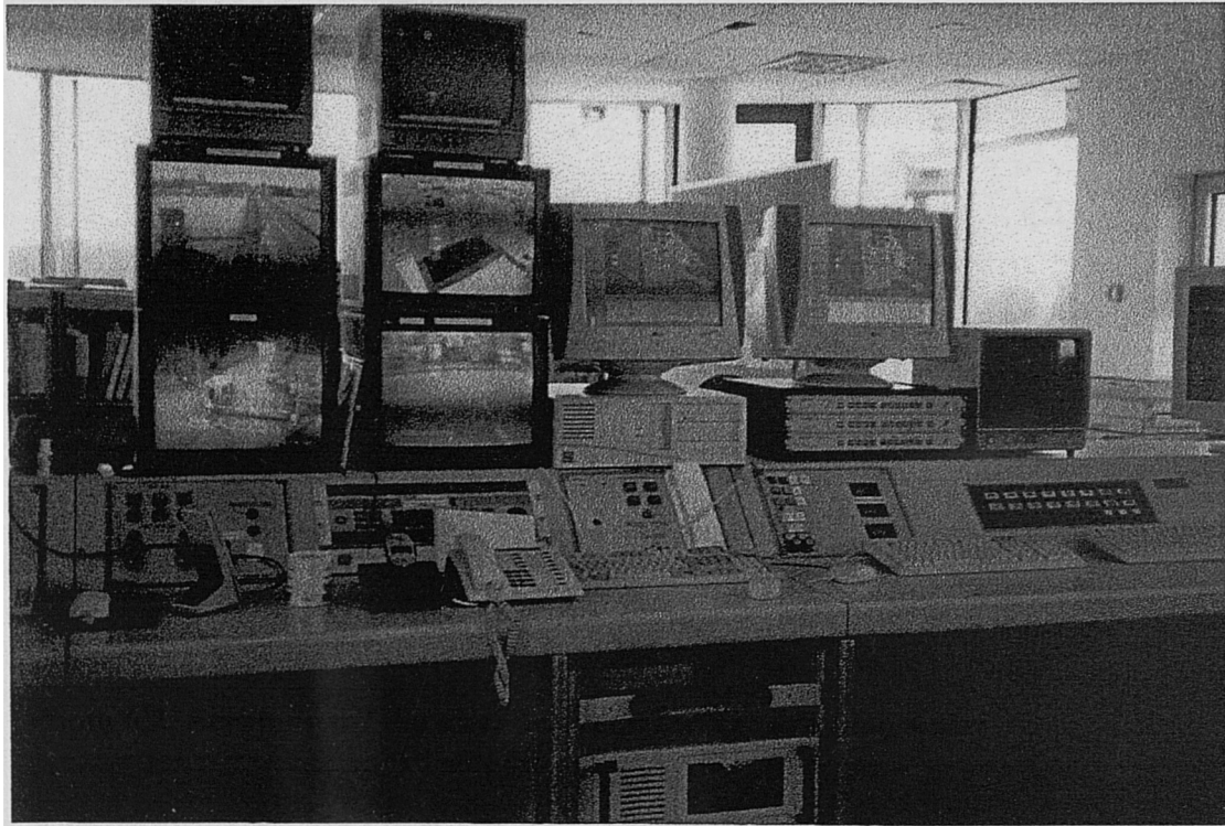
Photo 6.1: Entering the treatment plant: security and data information
