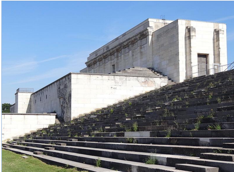
Figure 5. Speer’s decayed ‘bridge of tradition’, Zeppelinfeld, Nuremberg (2012).
