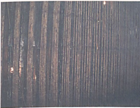
Figure 4.4 Superheater tube panels
