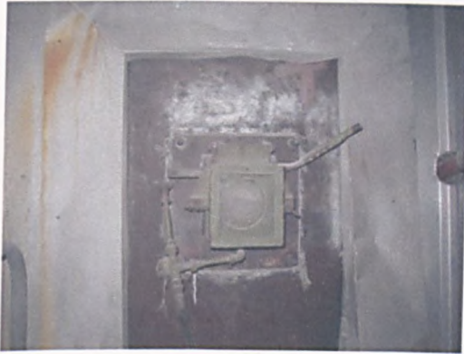
Figure 4.7 Viewing port at the location of probe No.1
