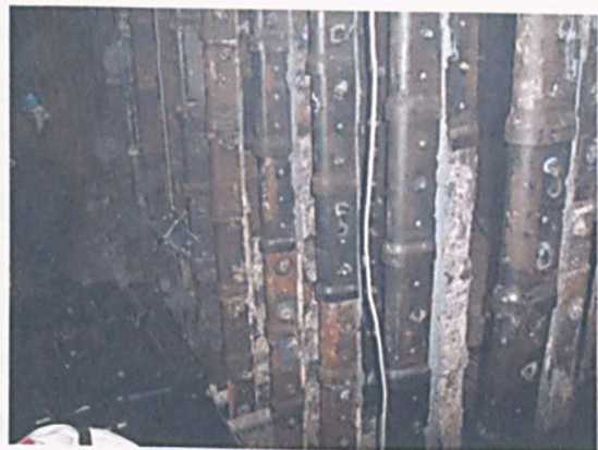
Figure 4.5 C-shape sacrificing shields encasing superheater tubes
