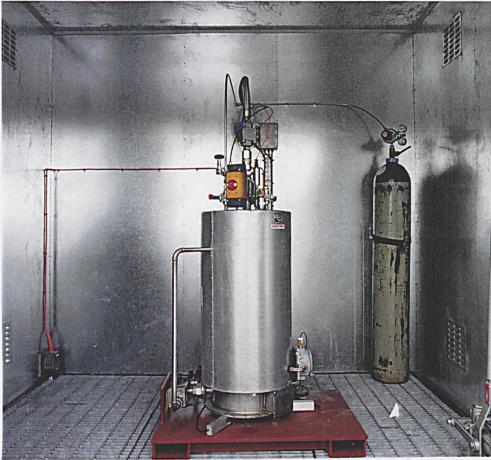
Figure 4.3 - Liquid Propane Storage Vessel
