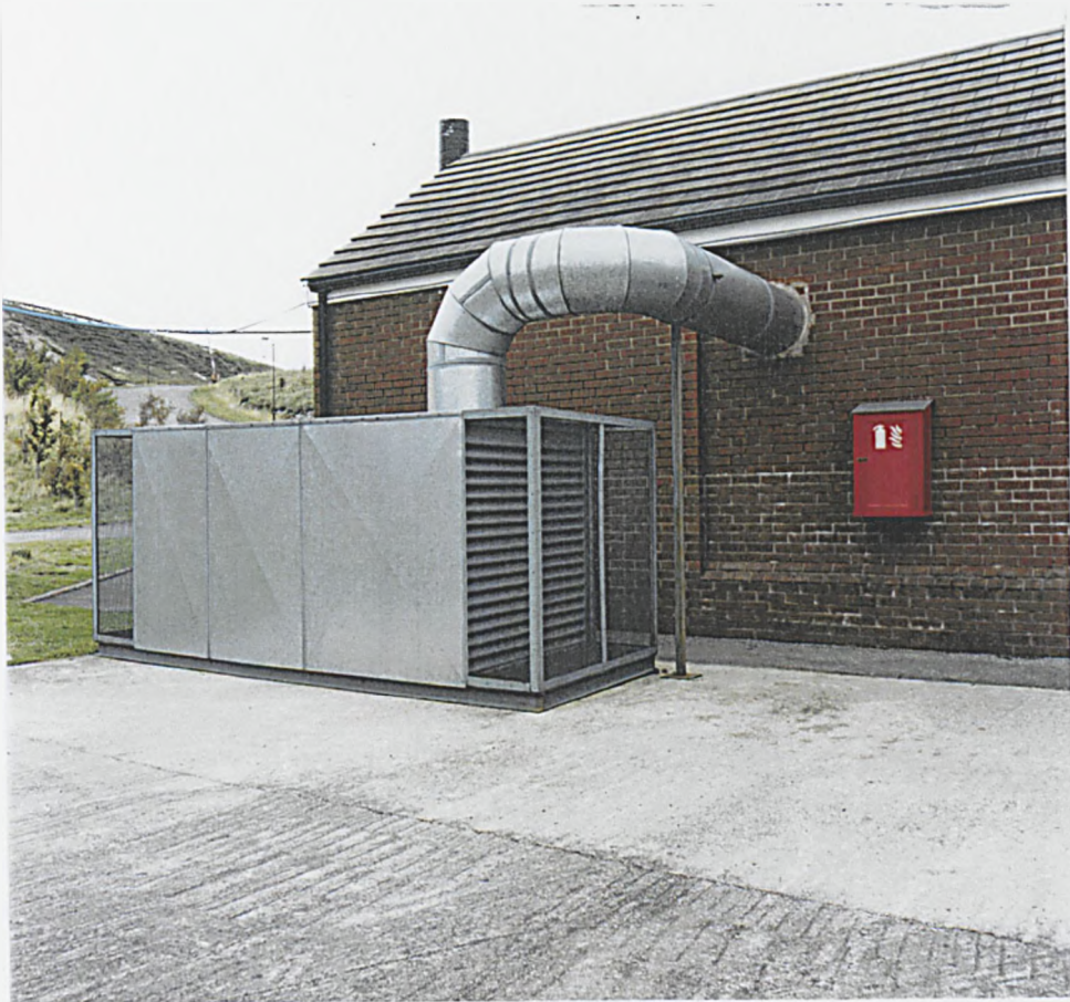
Figure 4.8 - Extract System Fan Unit
