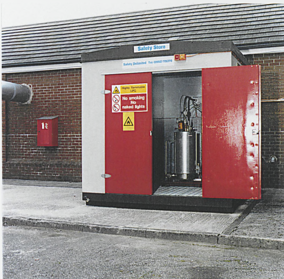
Figure 4.2 - Storage Vessel and Flameproof Store
