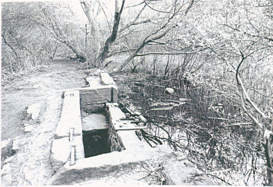
Figure 8a: Deep drain at Holme Head Wheel used when cleaning the dam to stop it from silting up. Note the slots in the masonry for the washboards used to raise the level of the dam and the top of the ratchet system used for raising the sluice.
