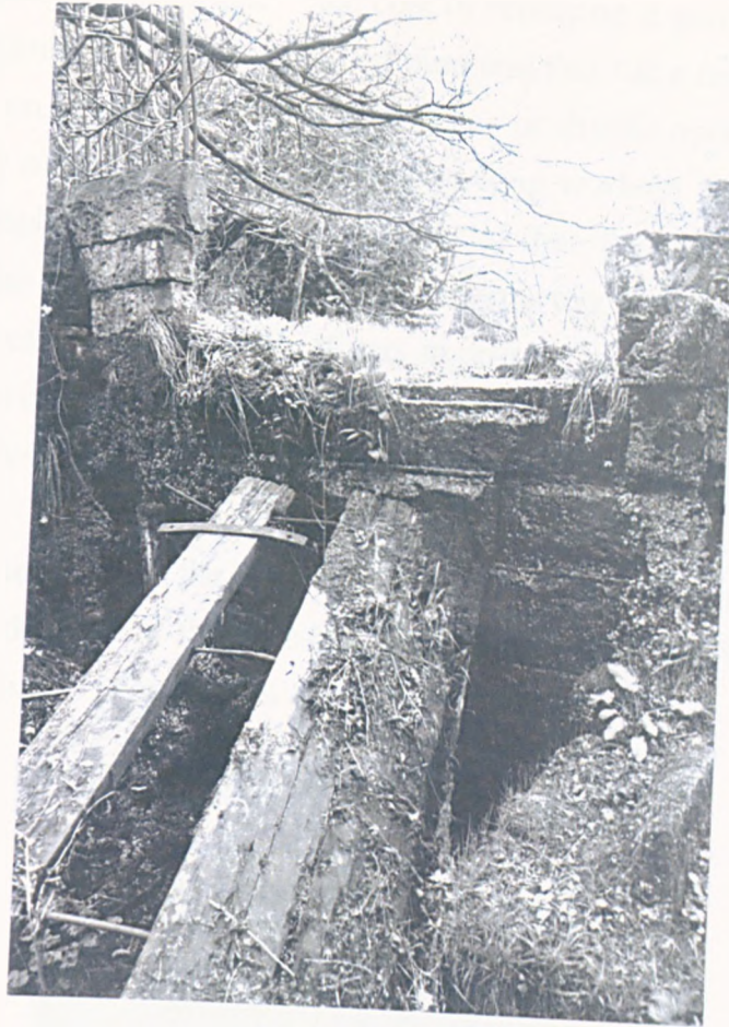
Figure 11b: Collapsed Pentrough at Holme Head Wheel looking towards the dam. (Rivelin)
