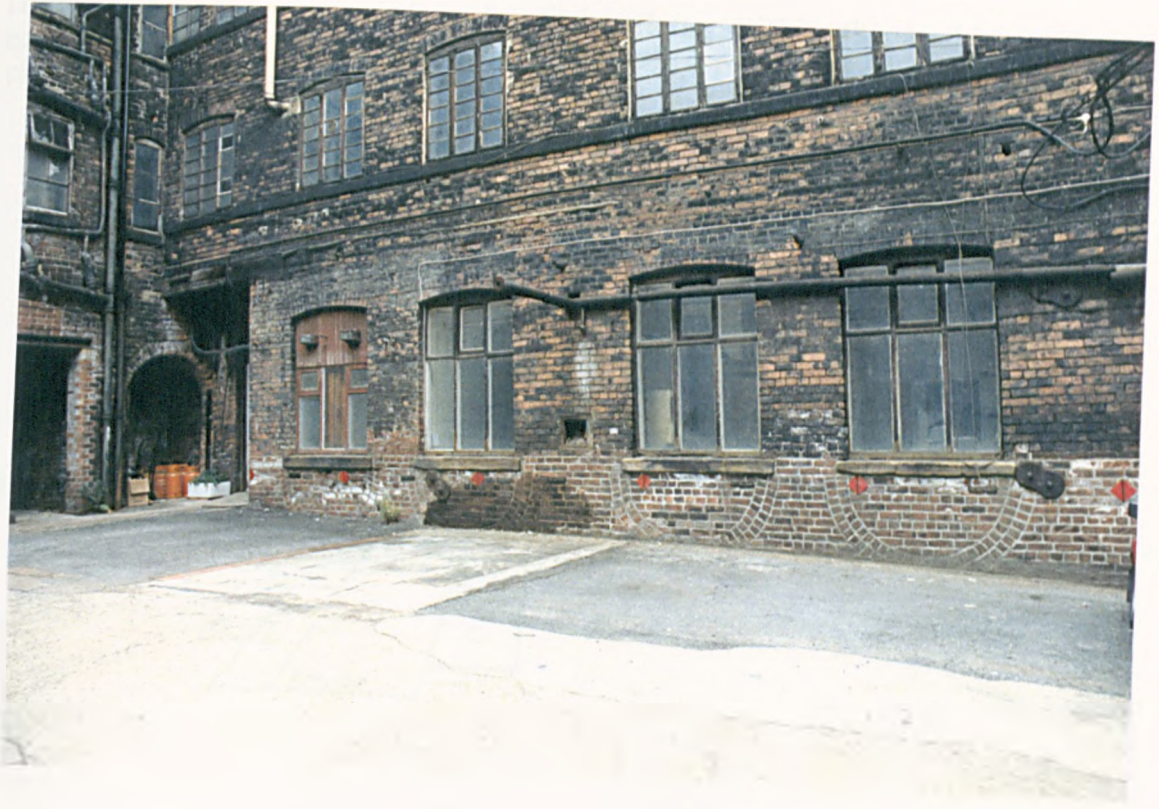
Figure 29b: Inverted arches in the courtyard to add strength to the original boiler room.
