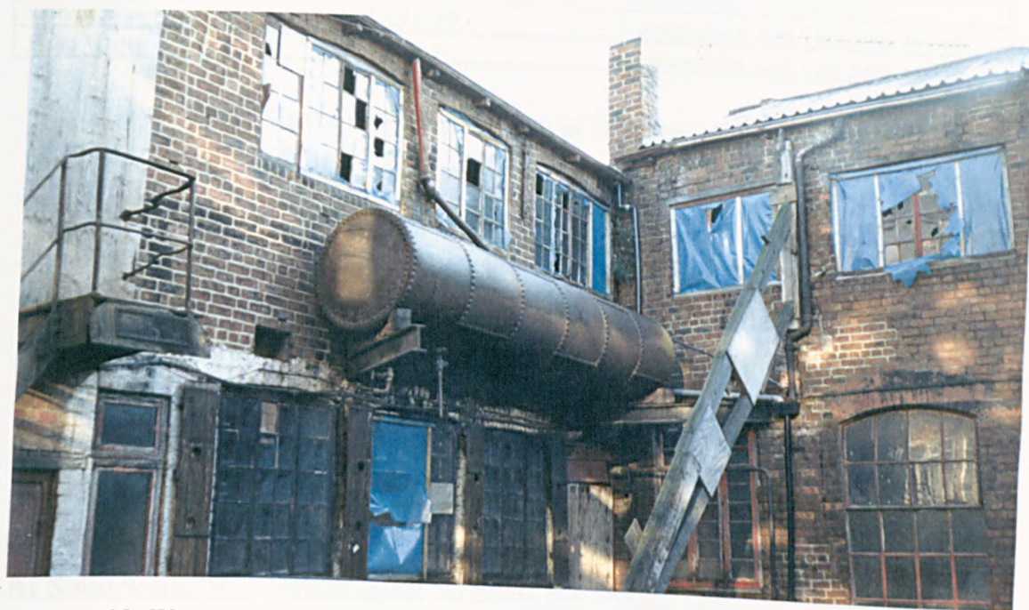
Figure 33: Water tank in Leah's Yard, Cambridge Street. The wagon boilers are located under the yard.
