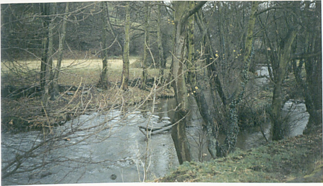
Figure 23b: Extended tail race at Rowell Bridge (Loxley) where remains of wooden piles either indicate the further extension of the bank or a system by which washboards were used to extend the length of the tail race.
