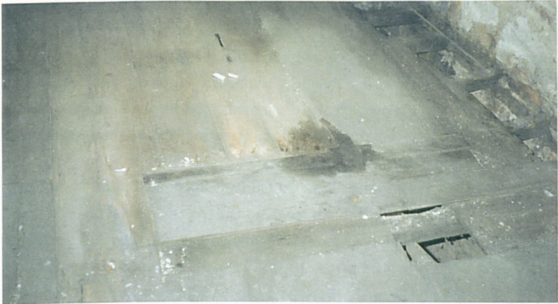
Figure 14: The floor at Kendal Works which has been patched many times.
