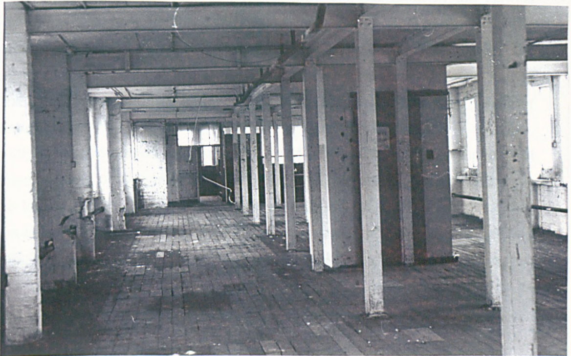
Figure 13b: The practice of reinforcing structures with metal beams was continued in the second floor packing house at Butcher's Wheel . Here, instead of cast iron, steel joists have been used.
