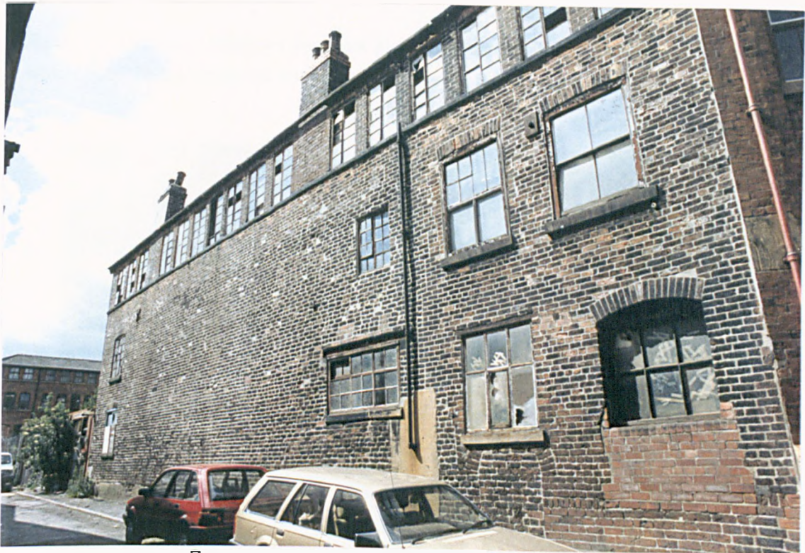
Figure 32b: “Low Shop” windows rarely survive. Here are some at Elliot’s, Sylvester Street, although not in their original form (A1). Again note the more typical windows above (B2).
