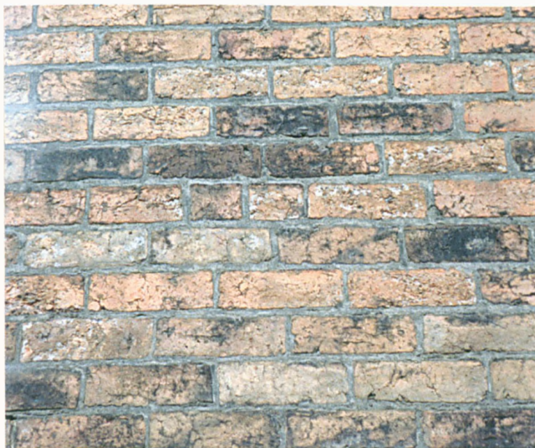
Figure 7i: Sheffield A Bond used in the construction of the Manager's Office at Eye Witness Works.
