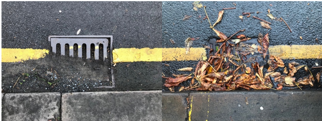
Figure 2-3 Conventional drainage clogged with sediments and leaves. Poor management of conventional system can cause severe floods.
