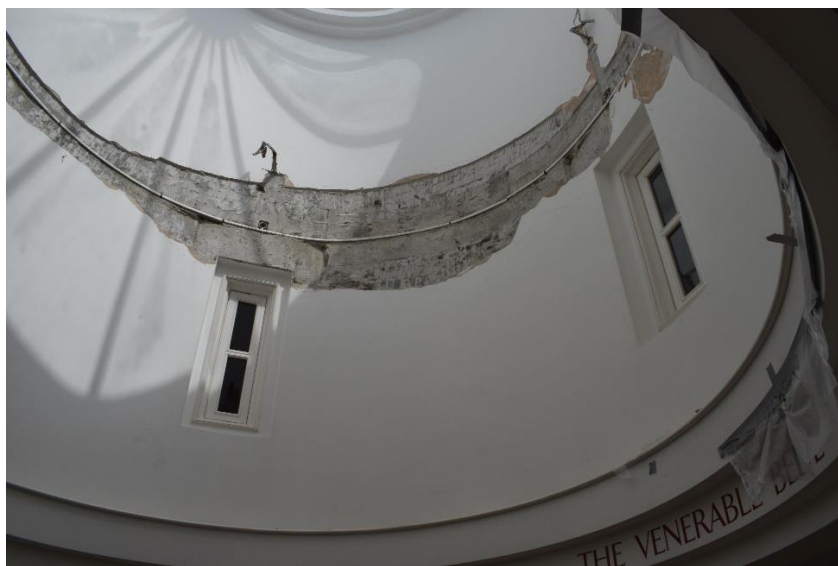
Damaged walls from the removal of the 'Mind of Bede' (2017) fig 7.42
