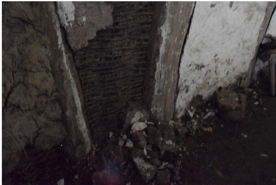
Collapsing interior of wattle and daub wall (2017) fig 5.53
