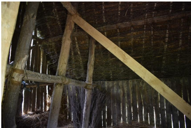
'The Oldest House' supported from collapse. West Stow, UK (2016) fig 3.5
