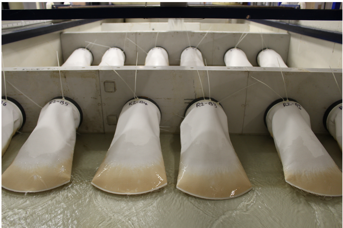
Figure 3.10: Picture of installed Filter Socks in ST01.
