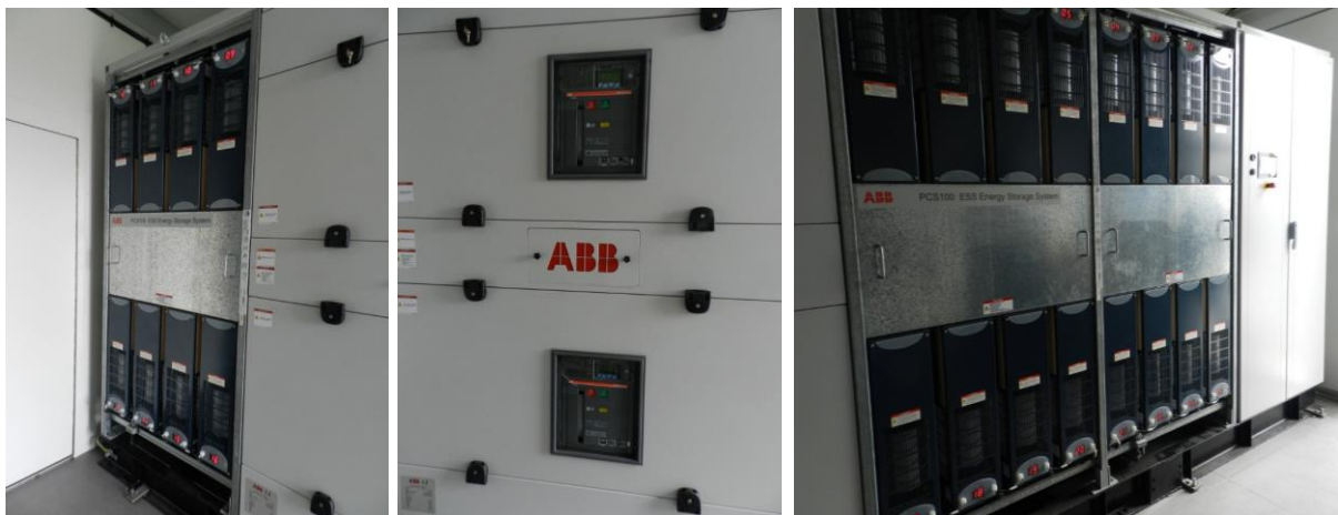
Fig. 4.6 Photos of 24 x ABB PCS100 converter in WESS.
