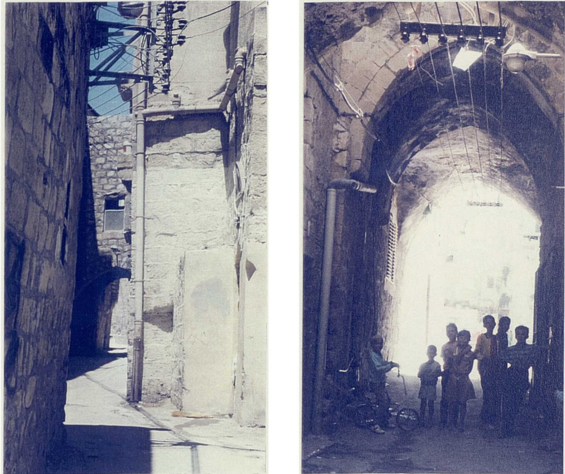
Fig. 7.18: Plastic Pipes Placed on Exterior Facades Damage the Street-scape of Old Nablus. Source: The Author
