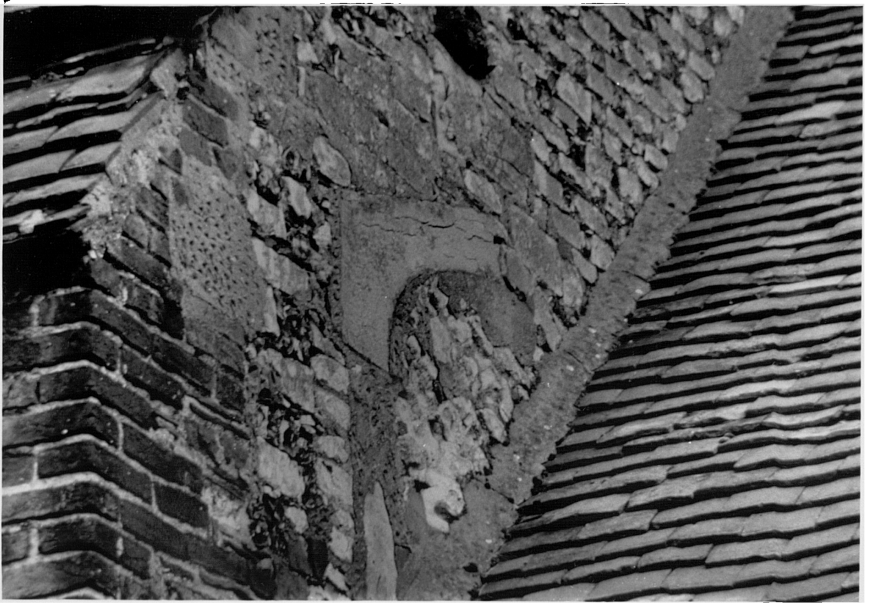
25 Blocked doorway from the east range to a gallery over the choir at Burnham (Berks).
