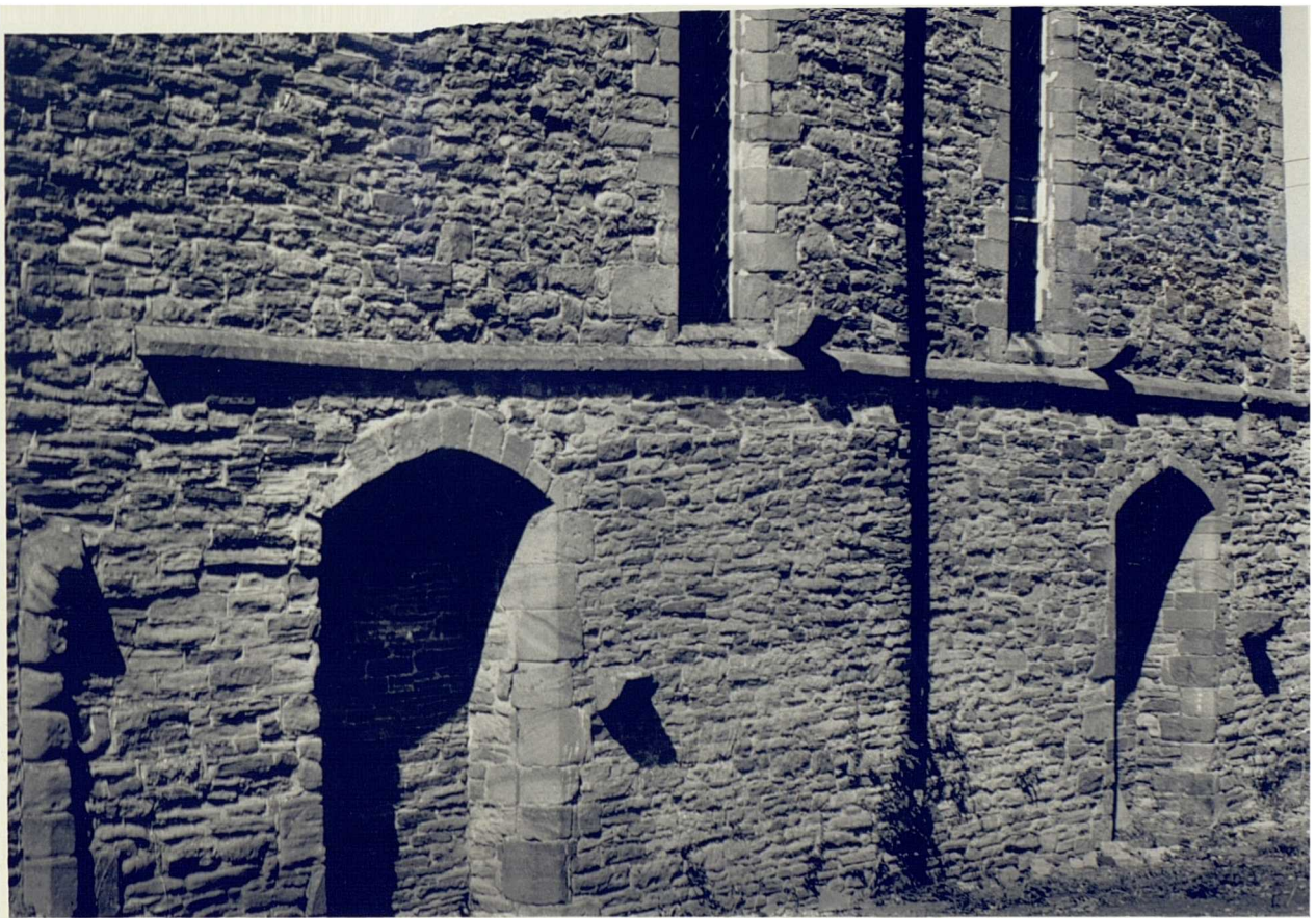
17 The south wall of the church at Aconbury (Herefords) retains corbel supports from the pentice roof of the cloister.
