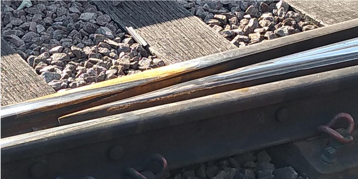
Figure 2-20 Crossing nose with fixed guiding (wing) rails at either side (Sheffield Train Station 2019)
