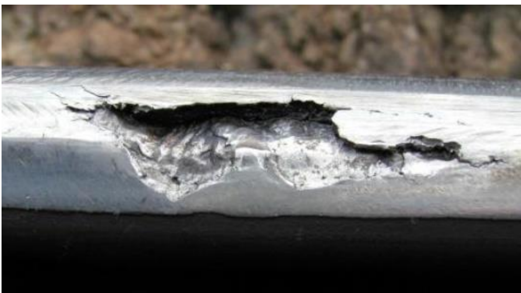
Figure 2-11 Shelling from gauge corner collapse [9]
