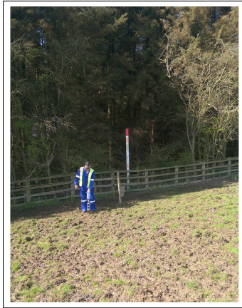
(a) Photograph of an operator using a pipe locator to place survey flags along the ground in the position above the centreline of the pipe.
