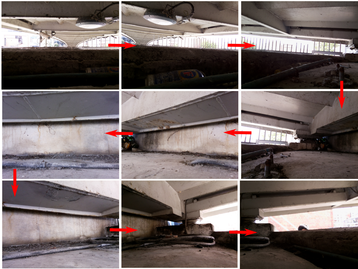
Figure 3.2: Photographs of the bridge bearing enclosure taken from on-board the robotic platform described in this Chapter. The arrows in the image show the sequence the photographs were taken in.
