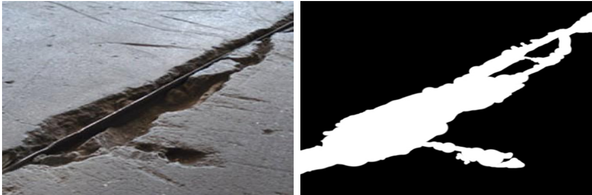
Figure 5.23: An example of an image and associated ground truth label in the CSSC dataset which contains a crack that has a high percentage of image pixels containing cracks.
