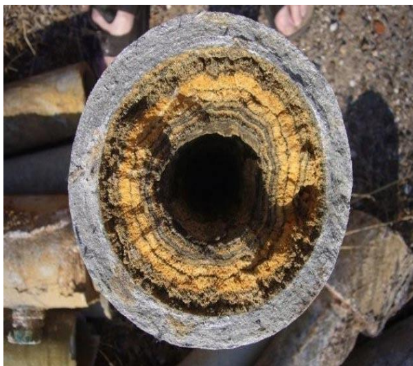
Figure 1-5 Blocking of a pipeline due to the growth of mineral scale [12]
