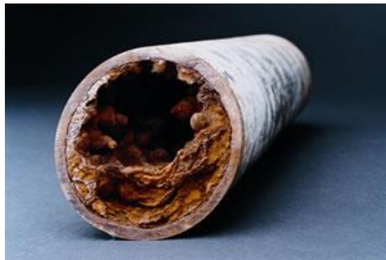
Figure 1-1 Scale deposition in a pipe [1]
