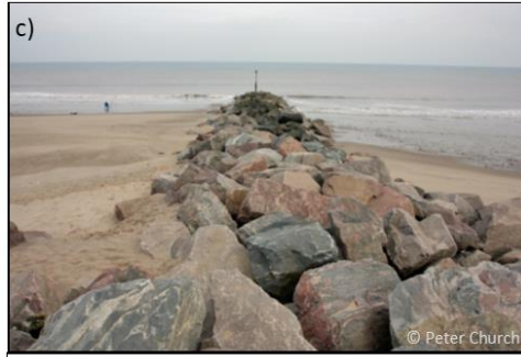
Rock groynes to encourage build-up of beach material and absorb wave energy
