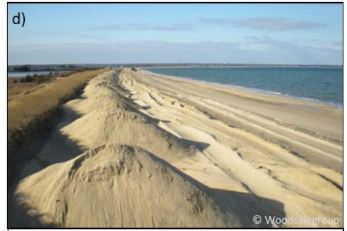
Beach "nourishment" through redistribution of sand, to replace lost beach material and help reduce erosion
