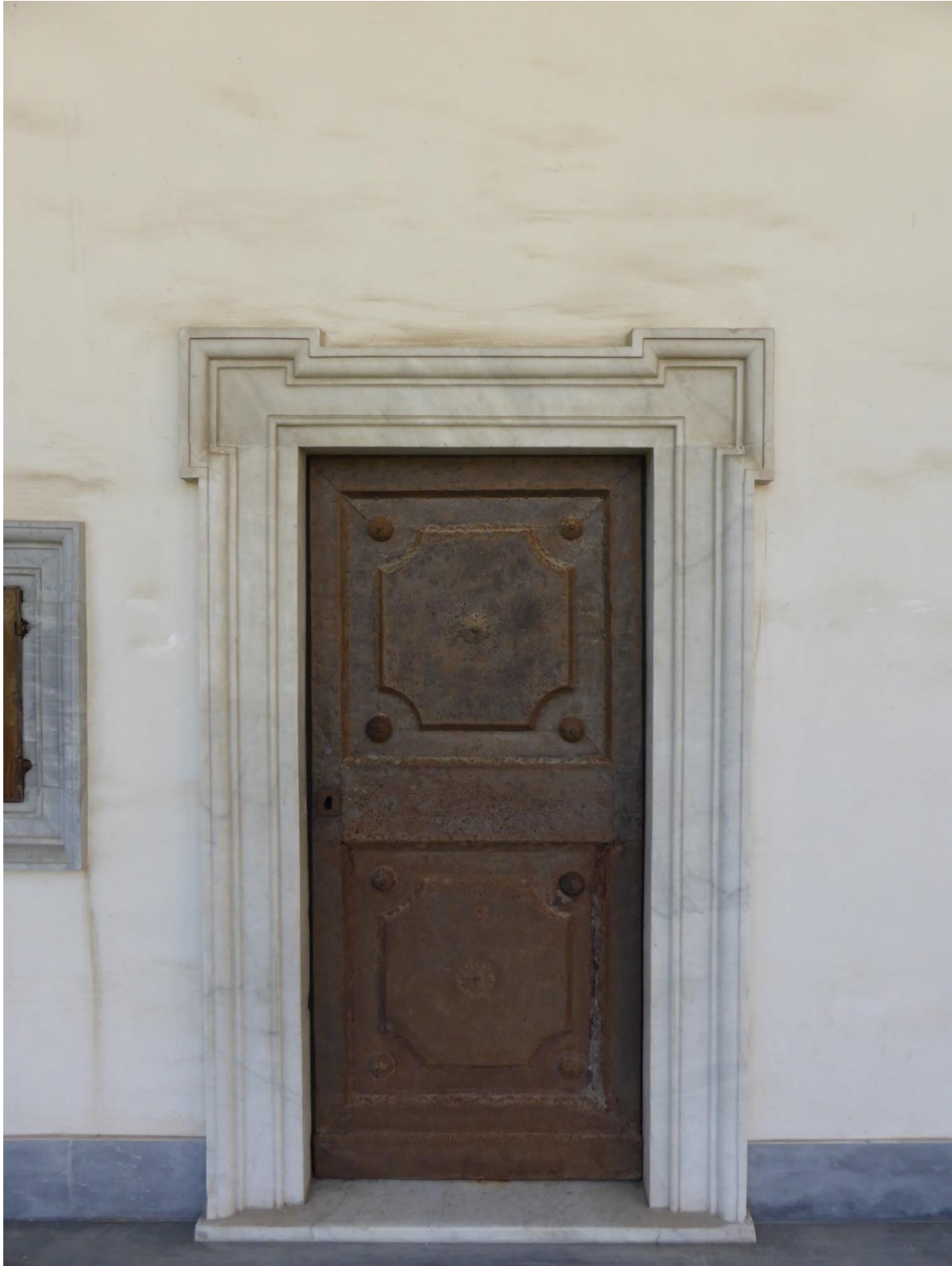
Figure 105: Great Cloister, Certosa di San Martino. Detail of individual cell door, with food hatch to the left. Source: author's own photograph.
