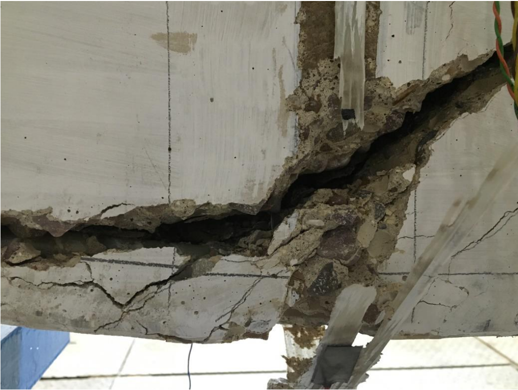
Photo 18 Shear link failure near shear crack (GB60)
