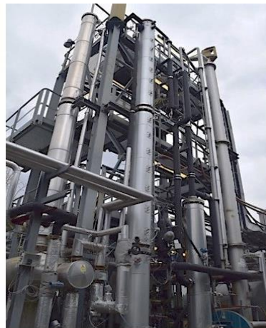
Figure 5.1. Photograph of the pilot-scale post-combustion CO 2 capture plant.
