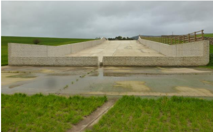
Figure 5.5: Eller Beck spillway channel from downstream with end sill at the front of the image
