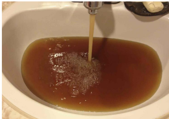
Figure 2.4. Discoloured water from a customer tap (Wazny, 2013).
