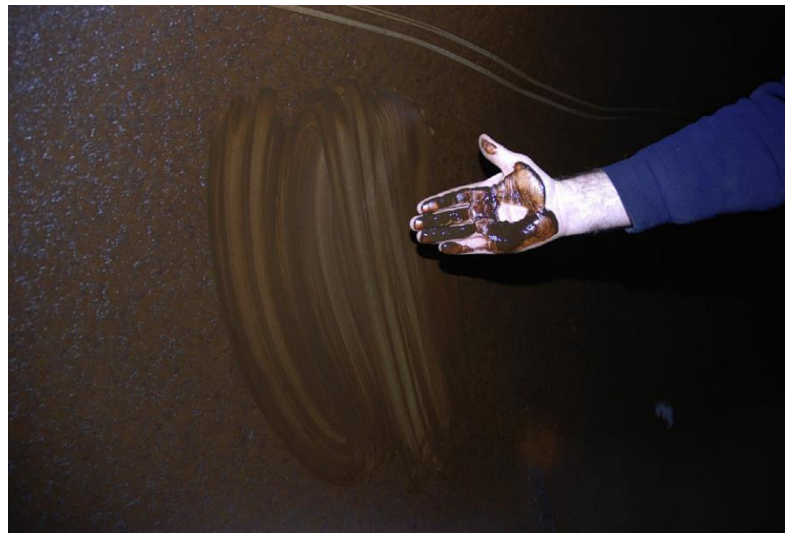
Figure 2.7. Photograph from inside a trunk main showing material adhesion across the internal pipe wall (Husband and Boxall, 2016).
