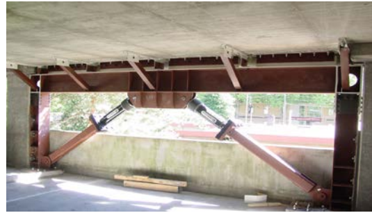
Fig.2.9 Viscous dampers in a parking garage [89]
