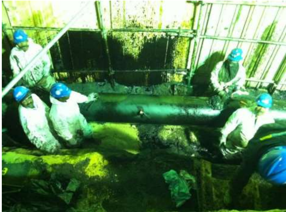
Figure 1-2: Leak due to internal corrosion in D-Filling line in South Tank Farm, Kuwait Oil Company (Original/Fieldwork).
