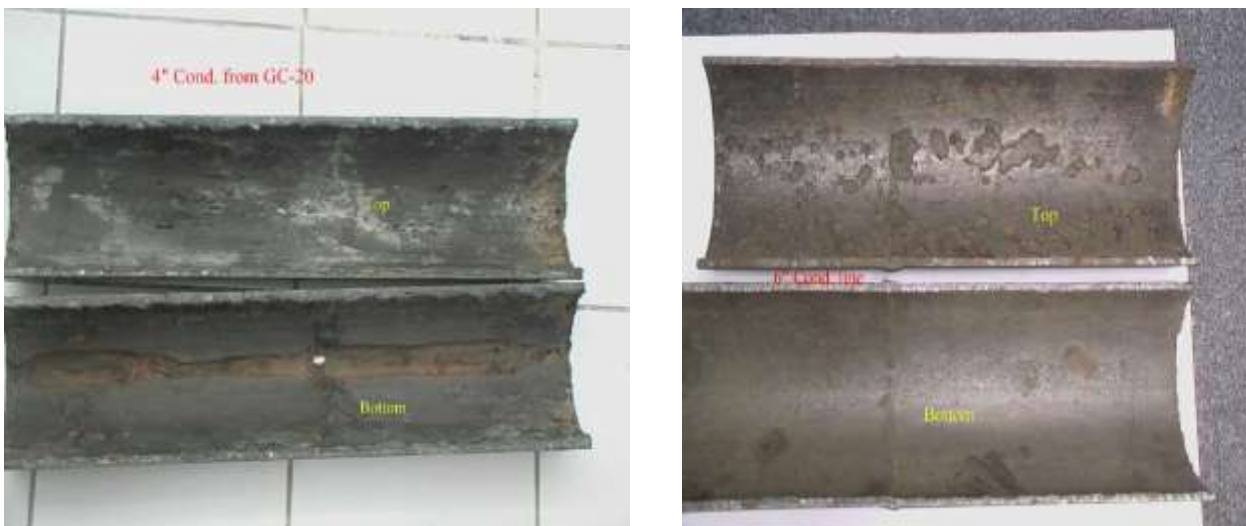
Figure 1-4: Corrosion in Condensate pipelines [6].
