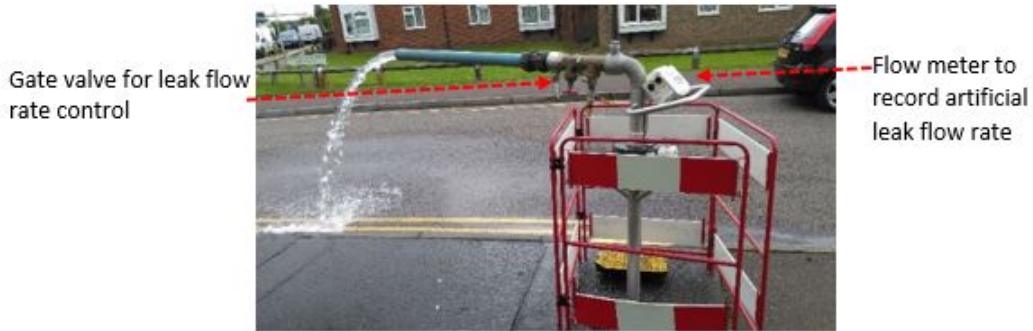
Figure 3.17: Standpipe with flow meter attached to fire hydrant on CI main. The same stand pipe and flow meter was used on all the pipe materials studied.
